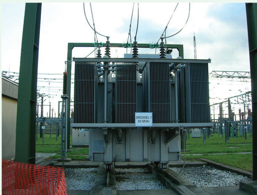
Figure TF26-1: A large 50 MVAR (Mega-Volts-Amps Reactive) loading inductor.
